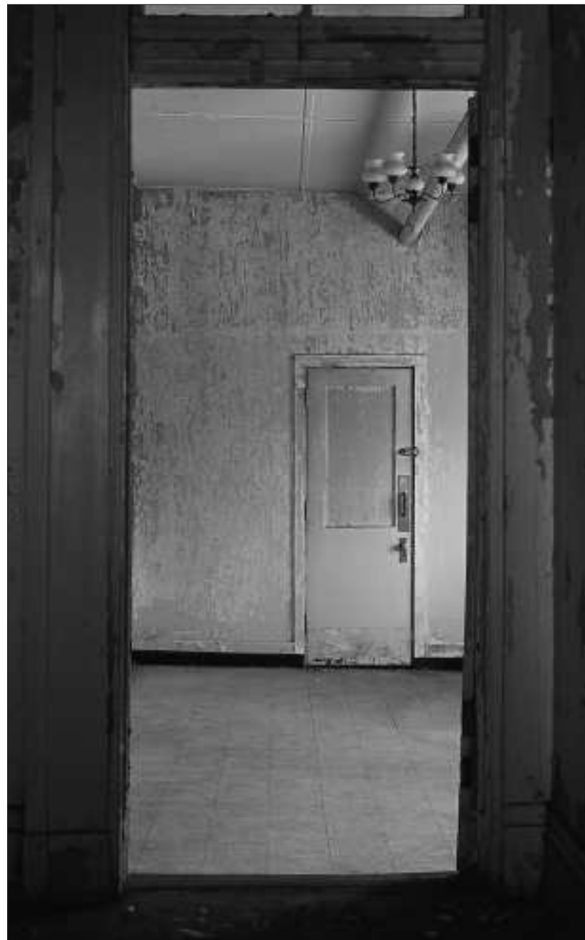
Changing the U.S. Marine Hospital’s status on the National Trust for Historic Preservation’s 11 Most Endangered list included among other tasks, peeling away the walls, doorways and windows that enclosed the original exterior galleries.
